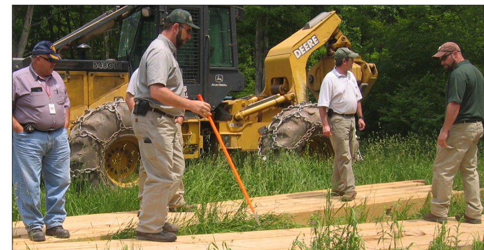
Common Waters offered a timber bridge workshop in early June. Portable timber bridge construction is one of four categories eligible for funding.
